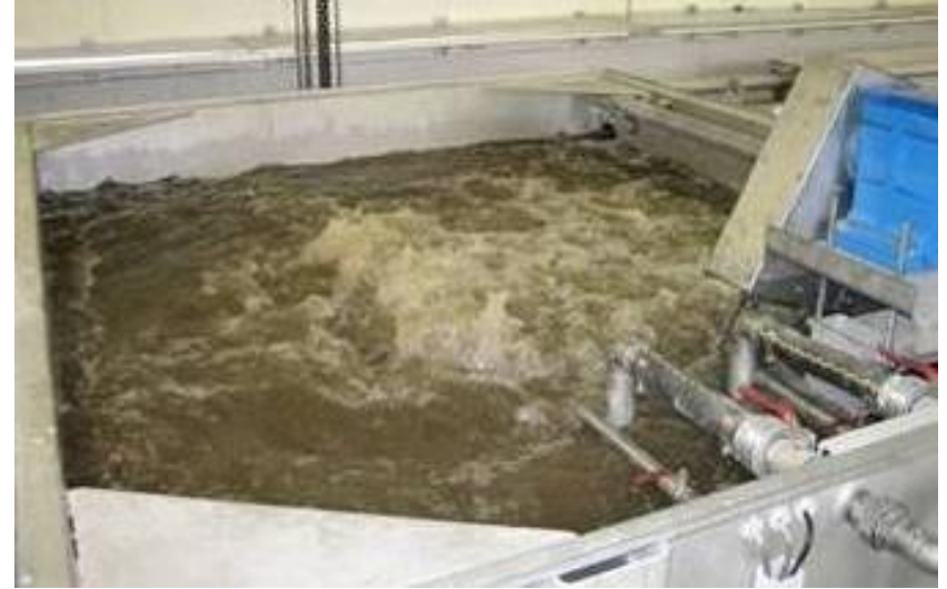
Filtration tank, HUBER BioMem® plant
