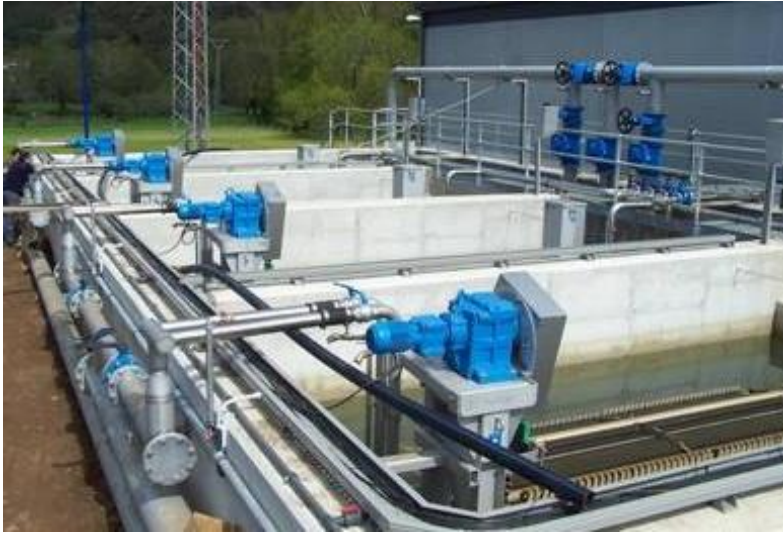
4 VRM® 30/448-Units in filtration chambers
