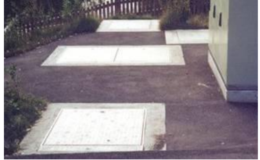
Manhole covers SD8: back-up proof, load-bearing
